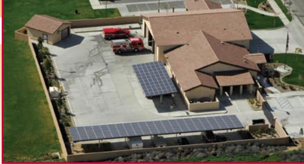
Solar panels, shown here at a Perris fire station, produce power most efficiently when they are oriented to capture as much sunlight as possible. The panels also create shade in hot areas.
